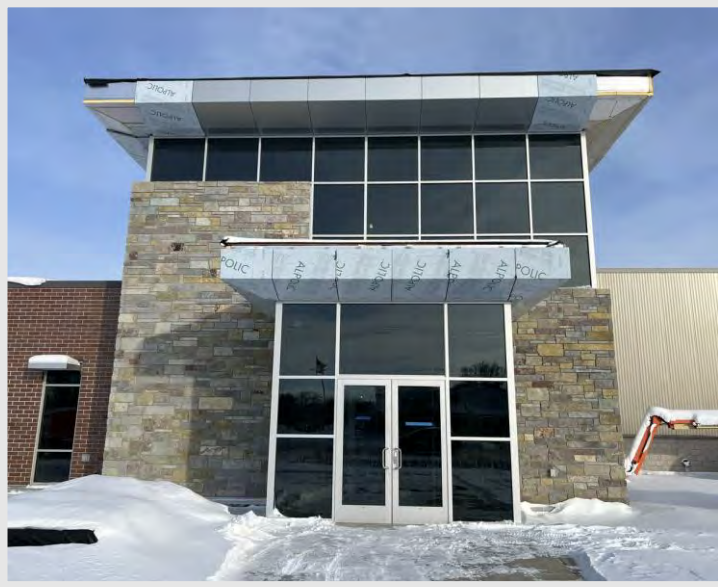
The aluminum storefront doors were installed at the front of the building, and soon the metal composite material panel install will complete.
