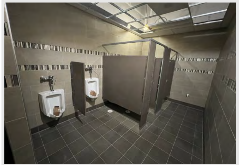
Findorff has installed the restroom partitions throughout the project in the previous week.
