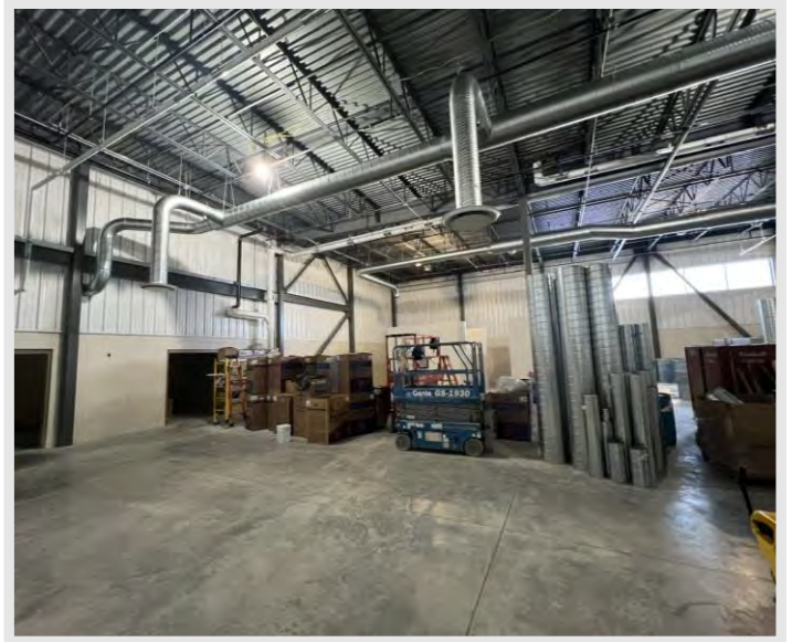
The mechanical, electrical, and plumbing installs are ongoing in the large lab spaces - pictured above is the Welding & Metal Fab. Lab.
