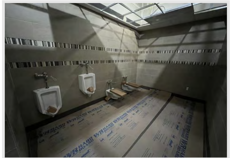
The restrooms have started to receive the plumbing fixtures throughout the building.
