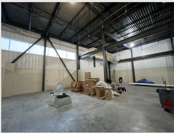
The sheets of white, interior metal liner panel has been installed above the CMU masonry walls throughout the labs.
