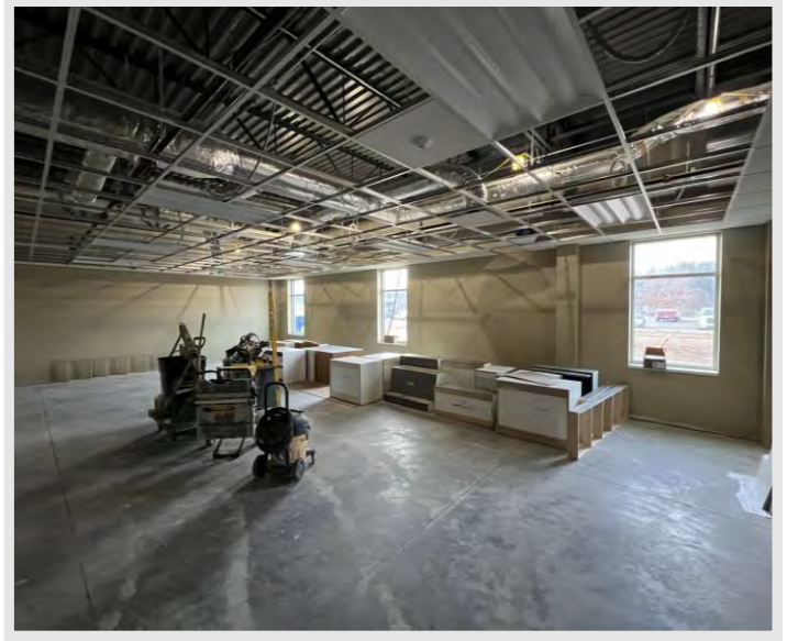
Casework was delivered to site and has been distributed throughout the site. Installation will occur in the coming weeks.
