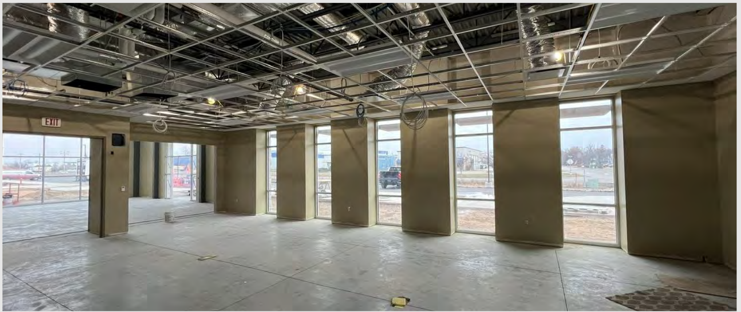
Above shows ceiling grid installed in the Community Room. You can also see that lay-in light fixtures are starting to be installed and connected by the electrician and the lay-in diffusers are being installed and connected to the ductwork systems by the mechanical contractor.
