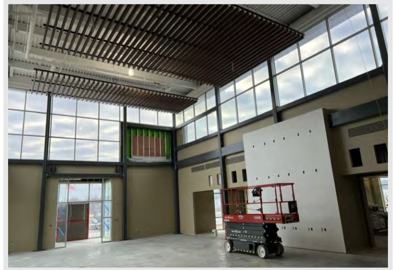
Notice the pre-engineered ceiling baffles that were installed in the atrium, they are supported from the metal decking above.
