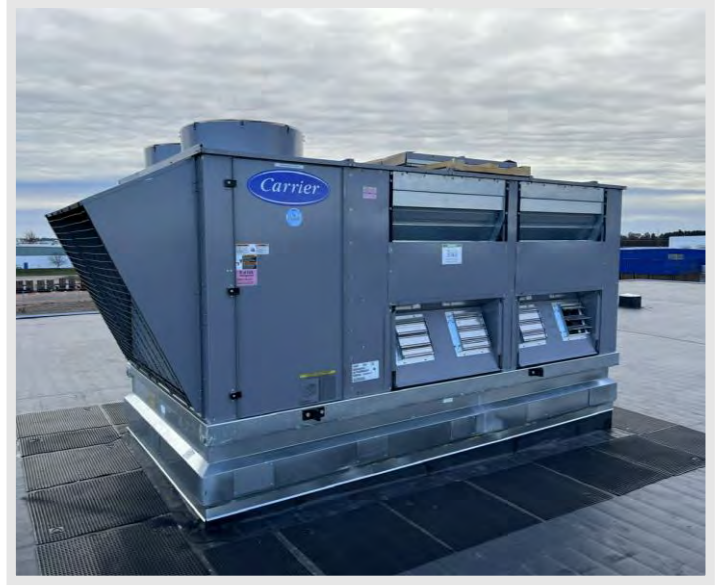
One of the six mechanical roof top unit's (RTU's) that was set into place on the roof via a crane in the past month.
