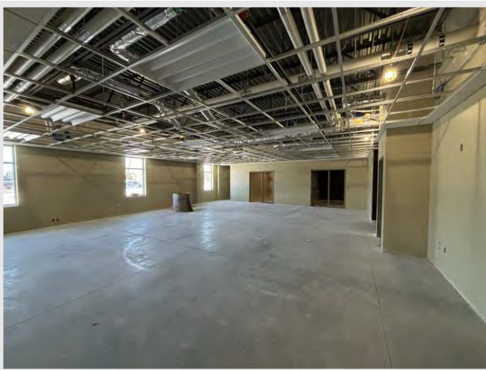
The ceiling grid install is underway in sequence one of the building and will continue in the coming weeks.
