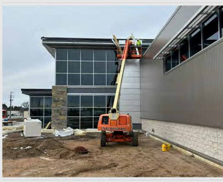
Insulation and metal composite material panel install continues to work around the main entrance area and upper atrium.
