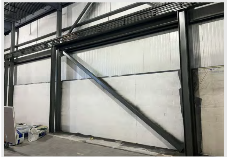
Painting of exposed steel has started in some areas around the building and painting will continue throughout the project.
