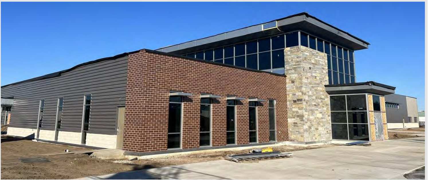
The masons have completed the stone veneer at the main entry and scaffolding has been removed as their demobilization takes place. Notice that metal composite material (MCM) panel installation has started at the upper atrium.
