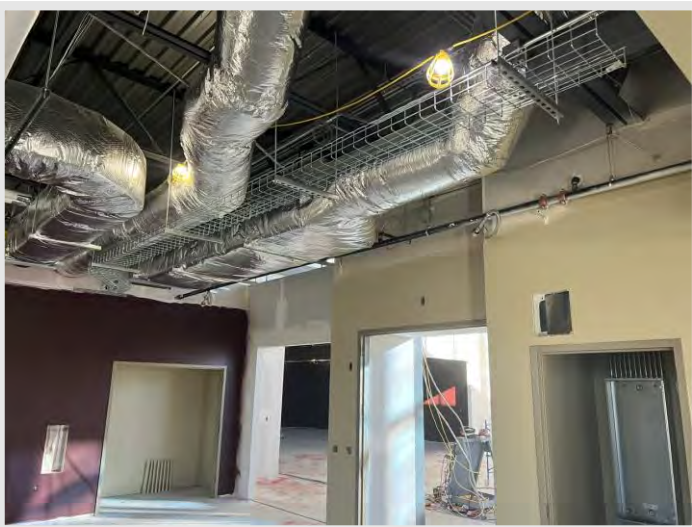
Ductwork is being insulated as work progresses and cable tray installation has kicked off in the past week.
