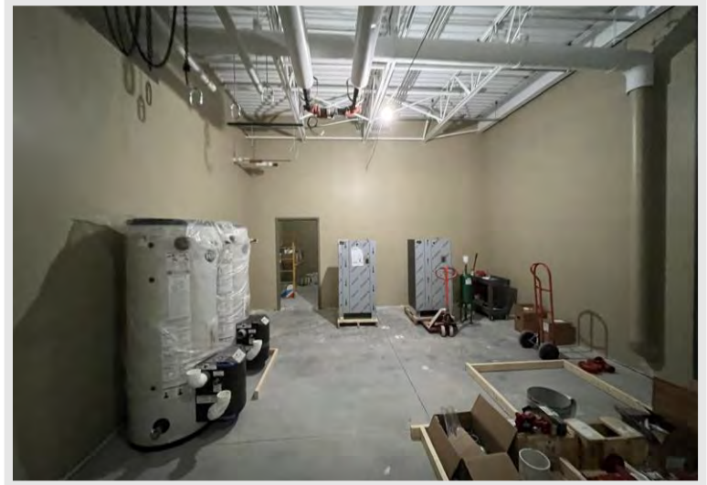
Some mechanical equipment is starting to be staged in 'back of house' spaces and we will see some equipment installs in the coming months.
