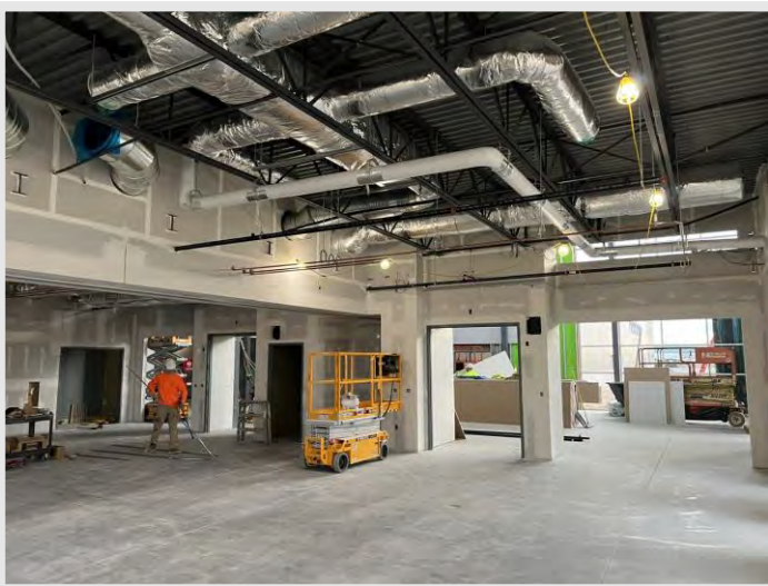
Mechanical, electrical, plumbing, and fire protection trade are finishing up sequence one of overhead installation, notice the systems in place.
