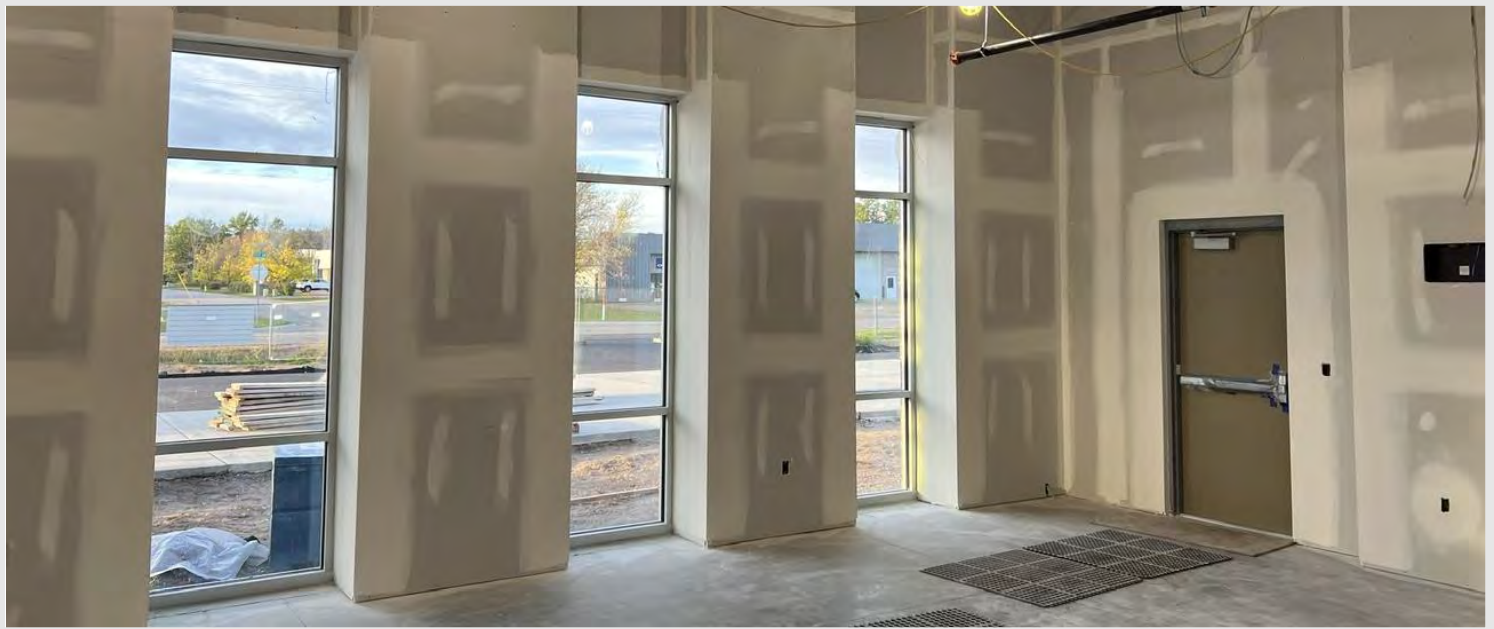
Sequence one awaits paint as all overhead mechanical, electrical, plumbing, and fire protection systems are in place and the drywall is taped, finished, and sanded. The lighter color area on the walls is drywall joint compound, which is used to conceal seams and screw heads from the install process.
