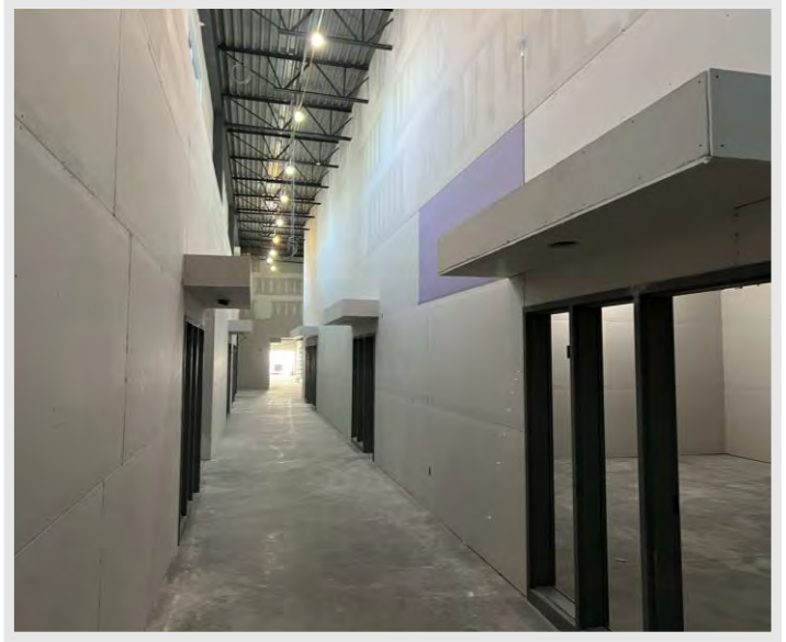
The soffits have been built and drywall has been hung in a central corridor of the building. Soon this area will be taped and finished.
