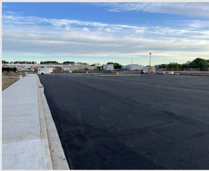
The remainder of asphalt binder course has been installed and the finish asphalt surface course is to be installed in the spring of 2024.
