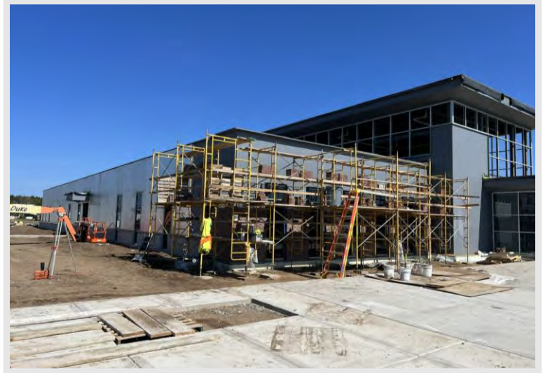
The masons have started the exterior brick and are utilizing scaffolding to work their way up the wall.
