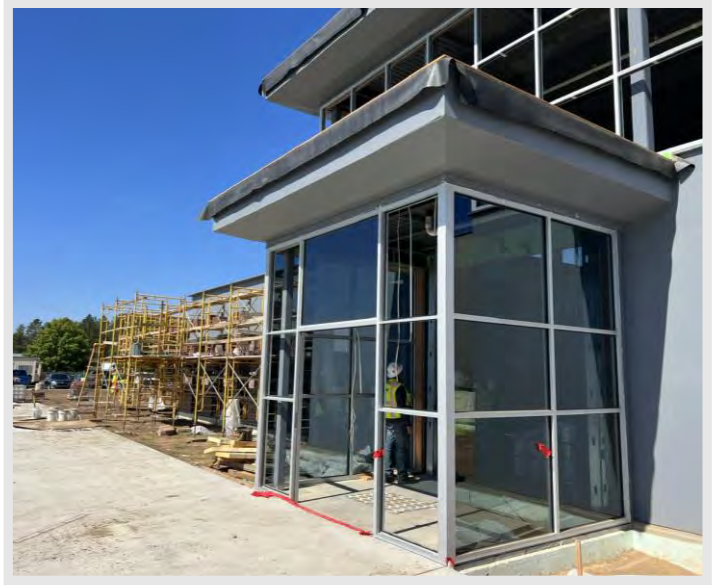
Aluminum storefront and glazing is occurring, and you can see the main entrance taking form in this photo!
