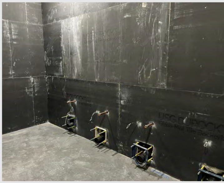
The west restrooms have received tile backerboard, which is water-resistant and used in wet areas like this, where future toilets will go.
