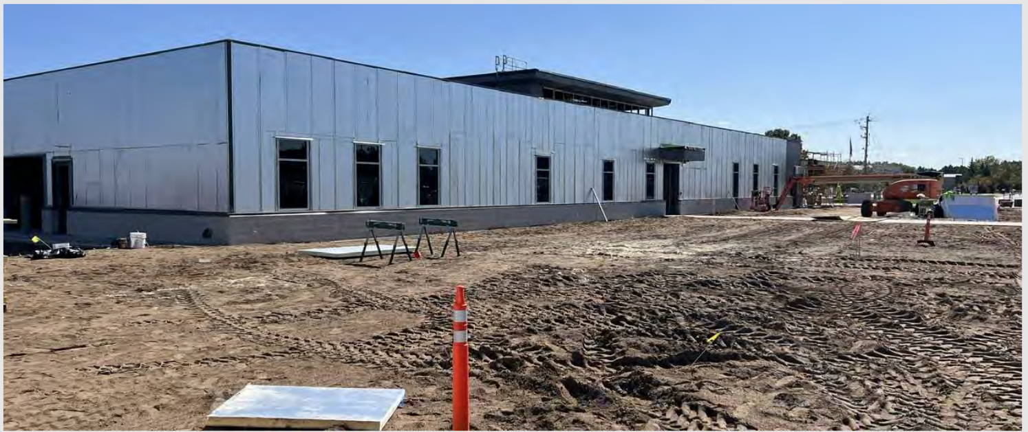
Foam board insulation is nearing completion at the west elevation and the north elevation. We will see metal panel being installed over these areas in the coming weeks, giving us a glimpse at the actual finishes of the building exterior.
