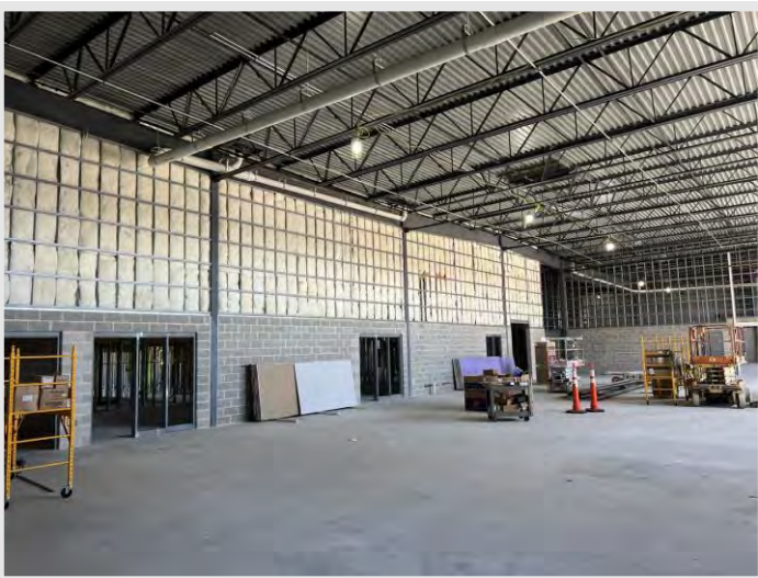
Insulation has been installed in some interior walls of future high-story lab areas.
