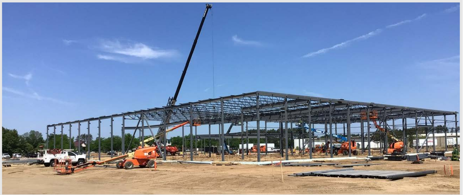
Overall view of structural steel installed shown from the Southeast corner of the building. Progress continues on the building as we look forward to having some of the enclosure trade partners coming to site in the coming weeks!
