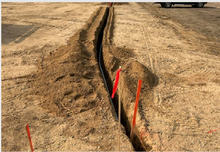
Site Electrical being trenched to the location of the future parking lot light poles.
