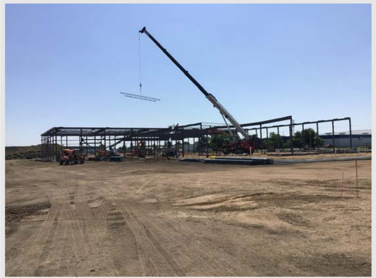
Rough Terrain Crane swinging joist into place. Each joist will be bolted and then welded as the building continues to go together
